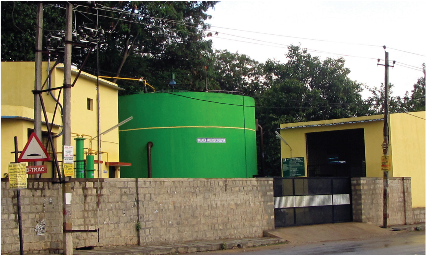
Mailhem's 5 MTPD biogas plant in Mathikere, Bengaluru
